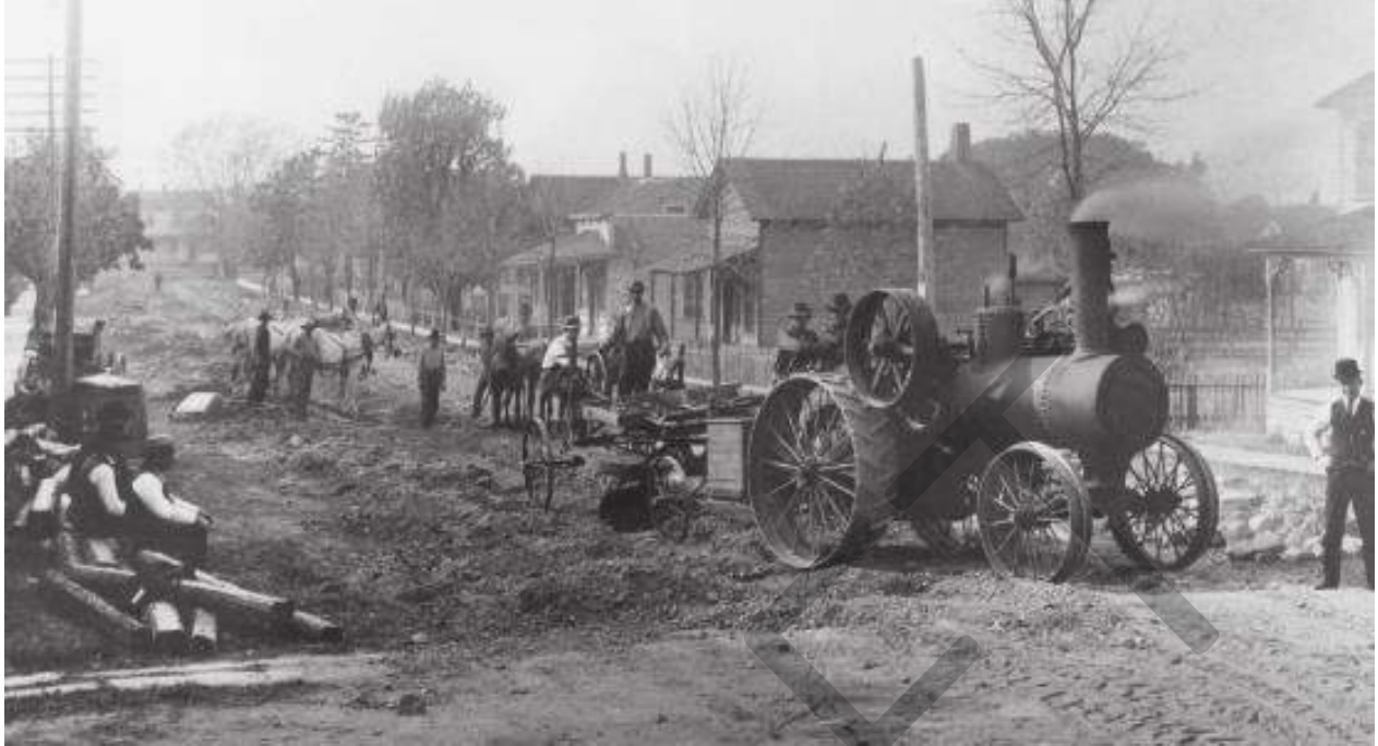
FIGURE 36: Photograph of track construction of the Joliet & Southern Traction Company extension from Aurora to Chicago Heights on Kansas Street in Frankfort, circa 1908. Source: Frankfort Area Historical Society.
